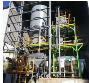
MBM Gasifier Plant 16 MWth steam. Oporto, Portugal
