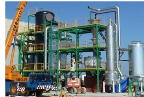
Wood chips Gasifier Plant 2 MWe CHP. Zaragoza, España
