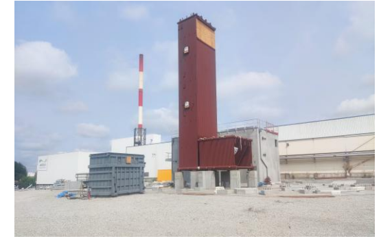
MBM Gasifier Plant 25 MWth steam. St Langis lès Mortagne France, Under Construction. Startup June 2025
