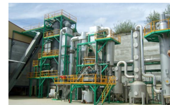
Wood chips Gasifier Plant 1.6 MWe CHP. Valencia, España
